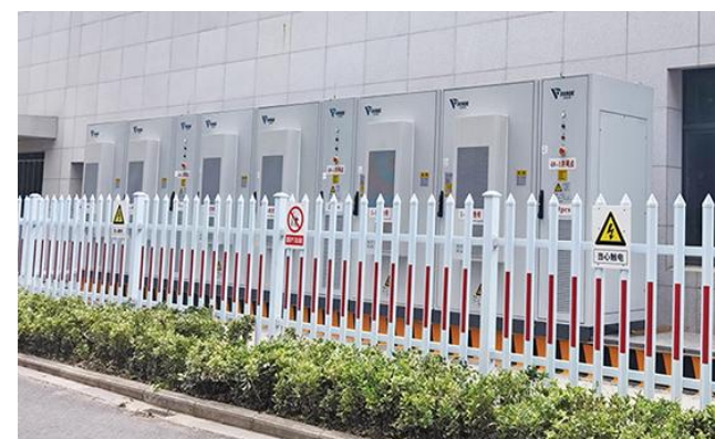
▲ JIANGSU NANTONG 3200kW/9890kWh Energy Storage Station
