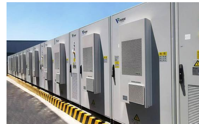
▲ JIANGSU HUAIAN 800kW/2580kWh Energy Storage Station
