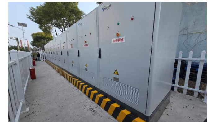
▲ JIANGSU HAIAN 1200kW/2580kWh Energy Storage Station
