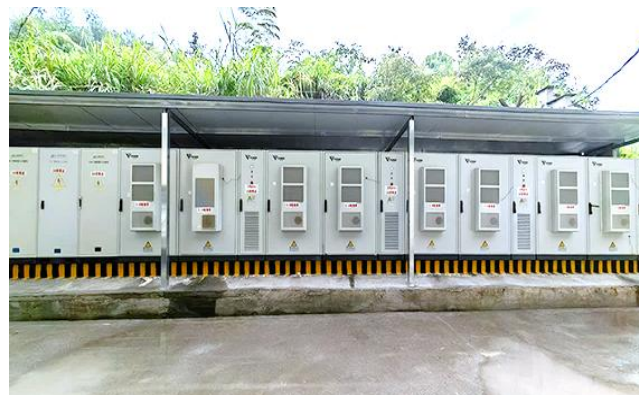
▲ ZHEJIANG LISHUI 900kW/1935kWh Energy Storage Station
