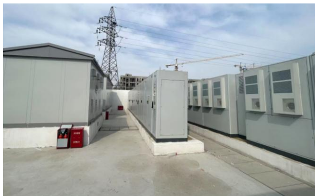
▲ JIANGSU SUQIAN 2148kW/6444kWh Energy Storage Station
