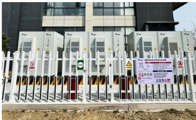
▲ JIANGSU YANCHENG 700kW/1505kWh Energy Storage Station
