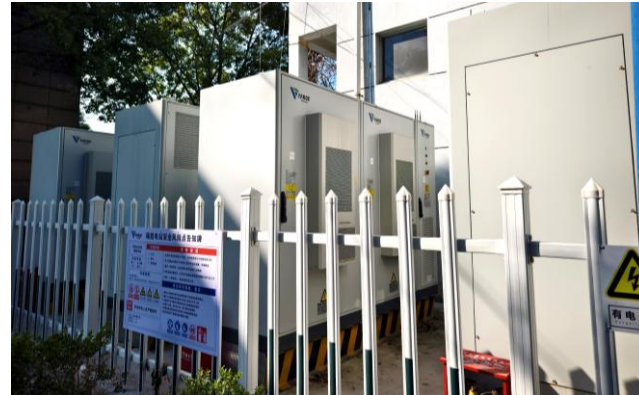
▲ JIANGSU HAIAN 900kW/2795kWh Energy Storage Station
