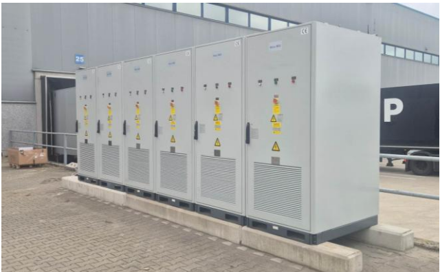
▲ NETHERLANDS 6*261kWh Energy Storage Station
