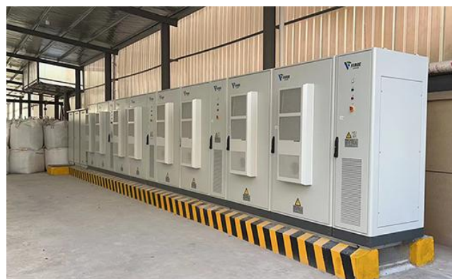
▲ ZHEJIANG JINHUA 800kW/1720kWh Energy Storage Station
