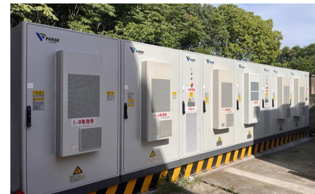
▲ JIANGSU SUZHOU 600kW/1720kWh Energy Storage Station
