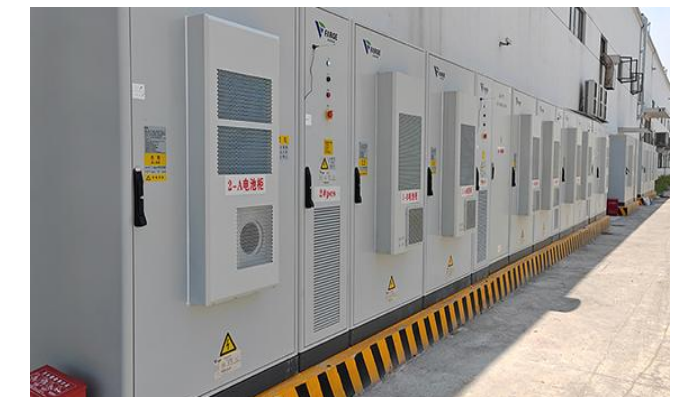
▲ ZHEJIANG HANGZHOU 1400kW/3010kWh Energy Storage Station
