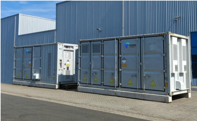
▲ NETHERLANDS 1260kW/2580kWh Energy Storage Station
