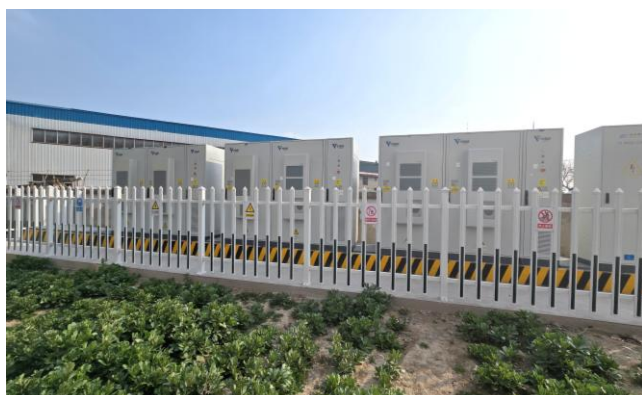
▲ JIANGSU HAIAN 600kW/1290kWh Energy Storage Station
