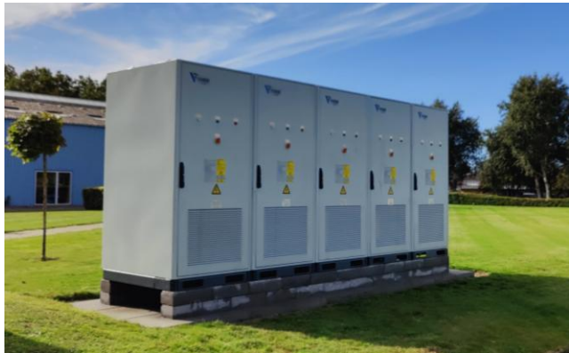
▲ DENMARK 5*261kWh Energy Storage Station
