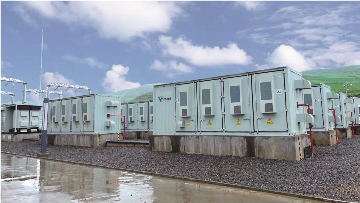
▲ GANSU GANNAN 9MW/18MWh Energy Storage Station
