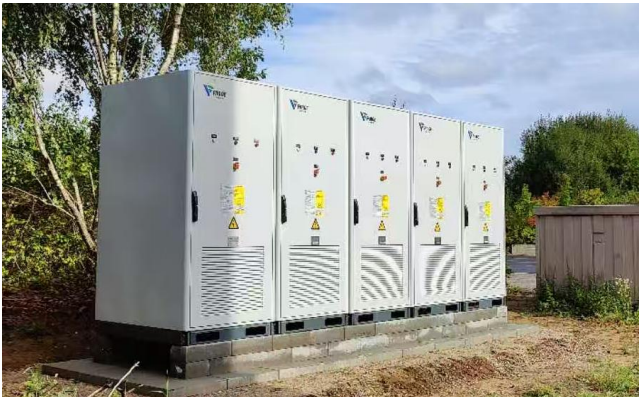
▲ DENMARK 5*261kWh Energy Storage Station
