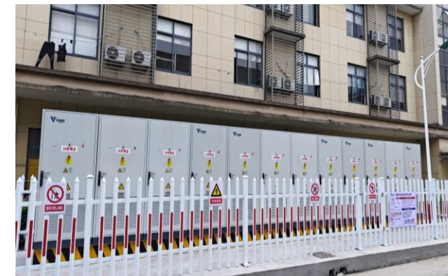
▲ ZHEJIANG JIAXING 1620kW/3132kWh Energy Storage Station
