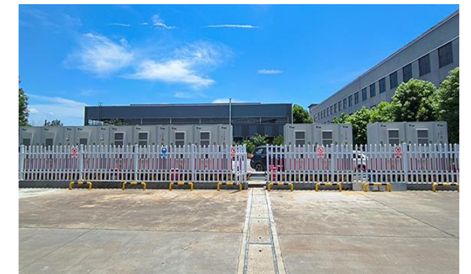
▲ ZHEJIANG ZHUJI 800kW/1720kWh Energy Storage Station
