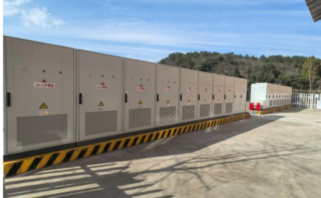
▲ ZHEJIANG ZHUJI 1992kW/5568kWh Energy Storage Station
