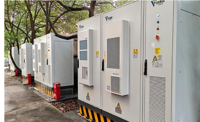
▲ ZHEJIANG JIAXING 2970kW/5805kWh Energy Storage Station
