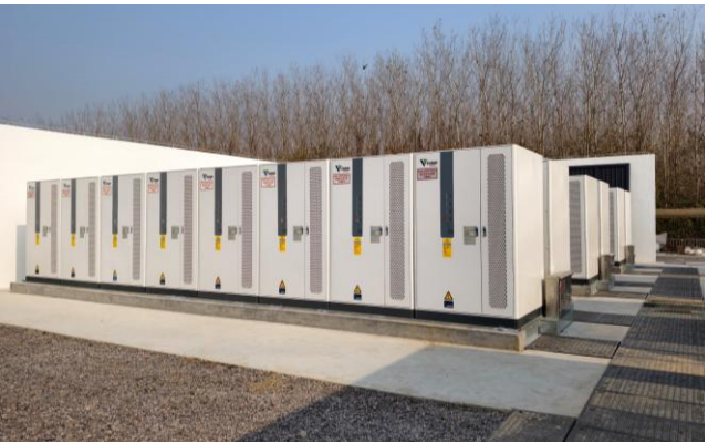
▲ JIANGSU NANTONG 9.45MW/20MWh Energy Storage Station
