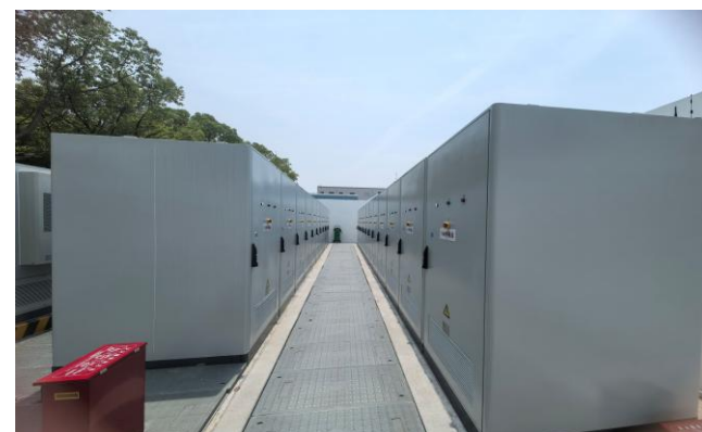
▲ JIANGSU HAIAN 5900kW/14219kWh Energy Storage Station
