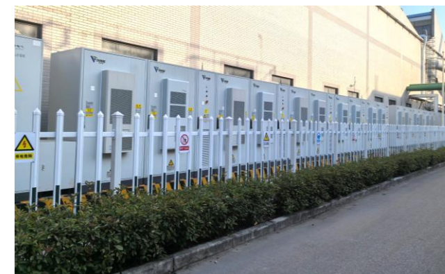
▲ JIANGSU NANTONG 1600kW/3440kWh Energy Storage Station
