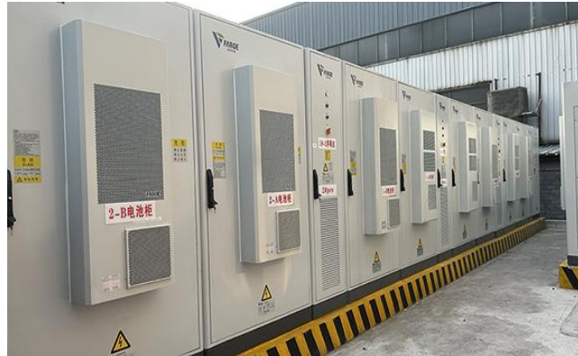
▲ ZHEJIANG HANGZHOU 1100kW/2365kWh Energy Storage Station
