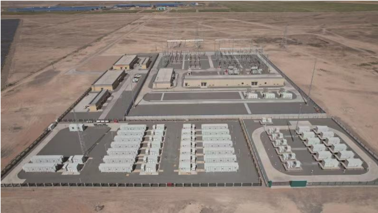
▲ GANSU JINCHANG 40MW/80MWh Energy Storage Station
