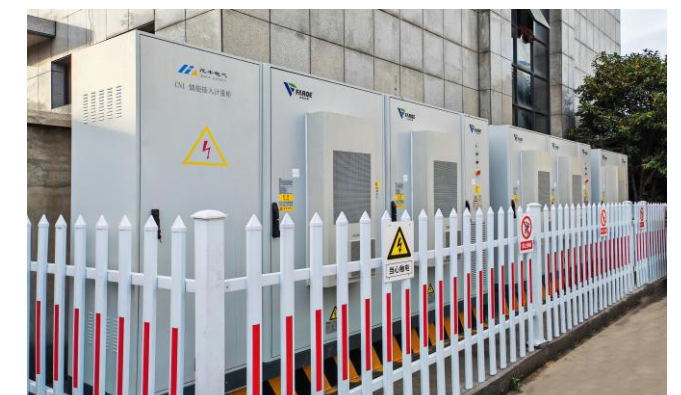
▲ ZHEJIANG HUZHOU 500kW/1075kWh Energy Storage Station
