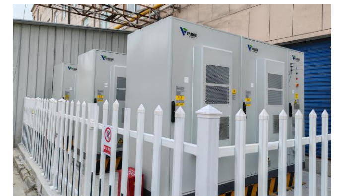
▲ JIANGSU JINTAN 1000kW/3010kWh Energy Storage Station
