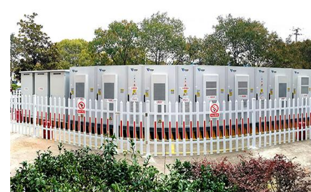
▲ JIANGSU NANTONG 700kW/1505kWh Energy Storage Station
