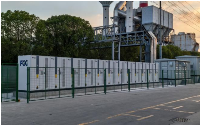
▲ ZHEJIANG JIAXING 4.9MW/9.614MWh Energy Storage Station
