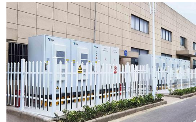
▲ JIANGSU NANTONG 800kW/2580kWh Energy Storage Station
