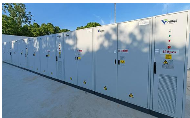
▲ JIANGSU KUNSHAN 5000kW/10750kWh Energy Storage Station
