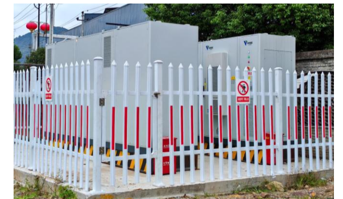
▲ ZHEJIANG HANGZHOU 600kW/1290kWh Energy Storage Station
