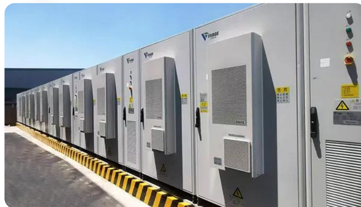
📍 Jiangsu Huaian 800kW/2580kWh
