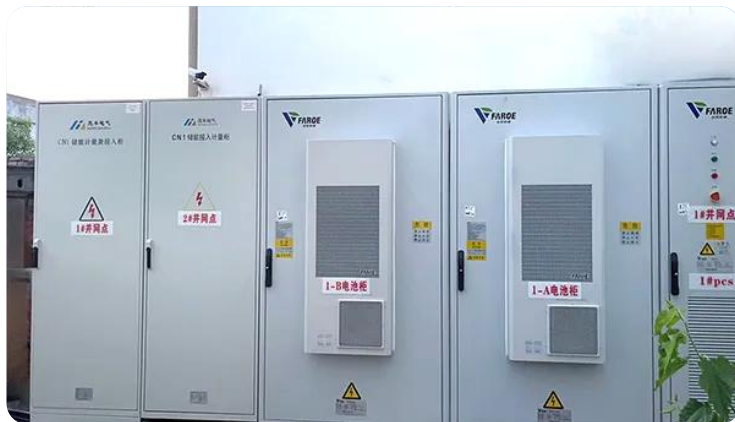
📍 Jiangsu Suzhou 400kW/1290kWh
