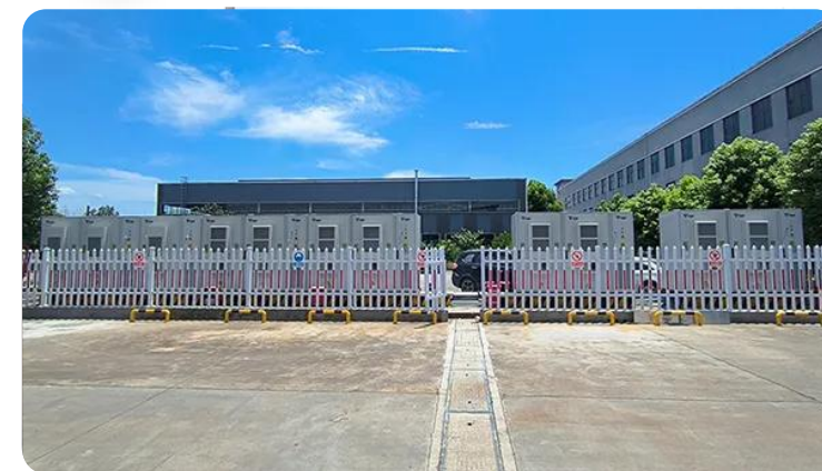
📍 Zhejiang Zhuji 800kW/1720kWh
