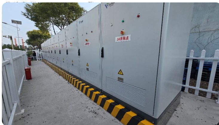
📍 Jiangsu Haian 1200kW/2580kWh
