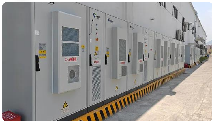
📍 Zhejiang Hangzhou 1400kW/3010kWh
