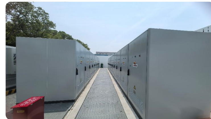
📍 Jiangsu Haian 5900kW/14219kWh
