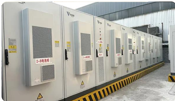
📍 Zhejiang Hangzhou 1100kW/2365kWh
