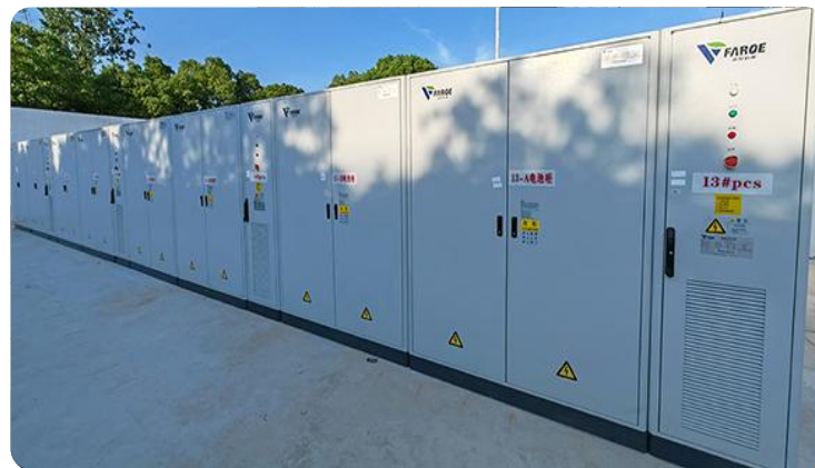
📍 Jiangsu Kunshan 5000kW/10750kWh
