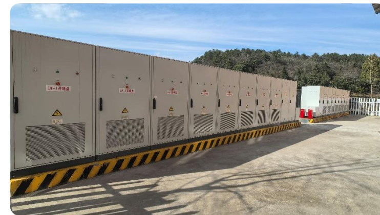
📍 Zhejiang Zhuji 1992kW/5568kWh
