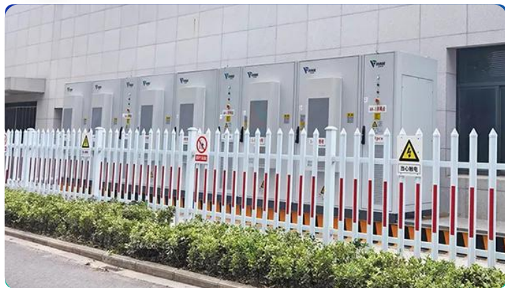
📍 Jiangsu Nantong 3200kW/9890kWh
