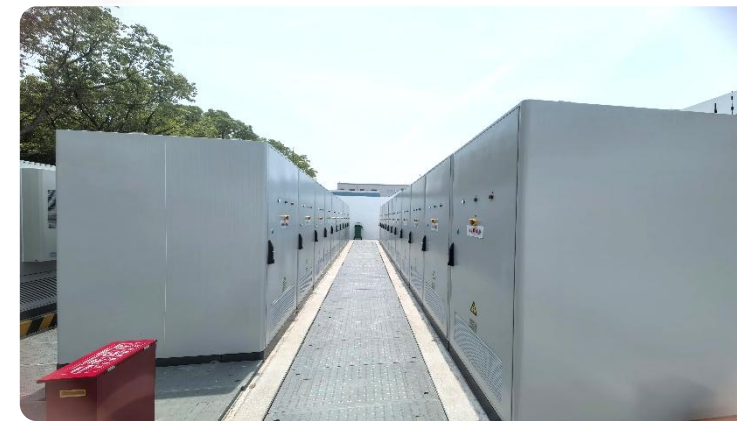
📍 Jiangsu Haian 5900kW/14219kWh
