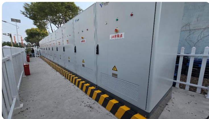
📍 Jiangsu Haian 1200kW/2580kWh
