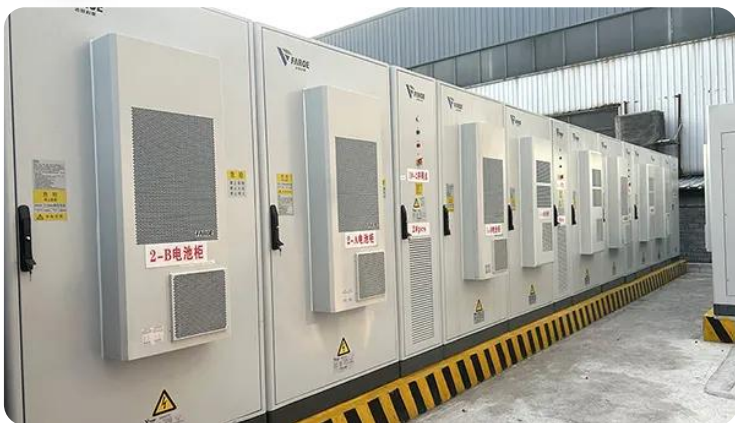
📍 Zhejiang Hangzhou 1100kW/2365kWh
