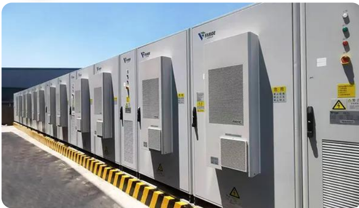
📍 Jiangsu Huaian 800kW/2580kWh
