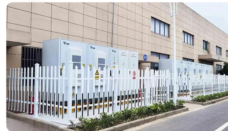
📍 Jiangsu Nantong 800kW/2580kWh
