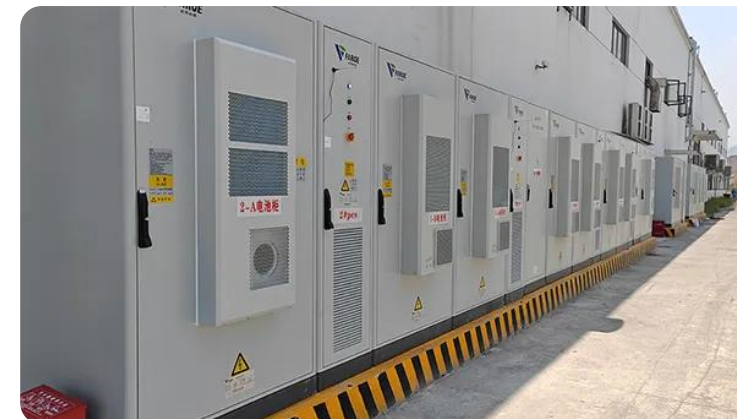
📍 Zhejiang Hangzhou 1400kW/3010kWh
