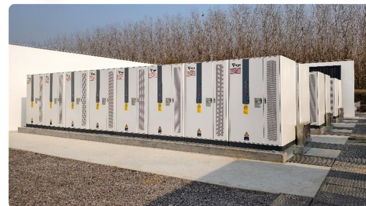
📍 Jiangsu Nantong 9.45MW/20MWh
