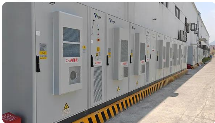
📍 Zhejiang Hangzhou 1400kW/3010kWh
