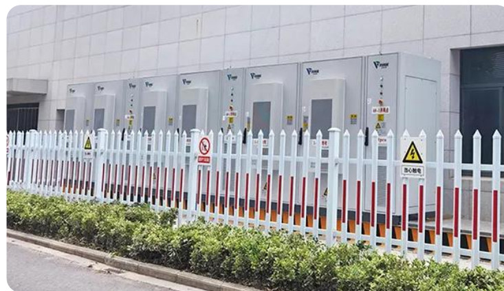
📍 Jiangsu Nantong 3200kW/9890KWh
