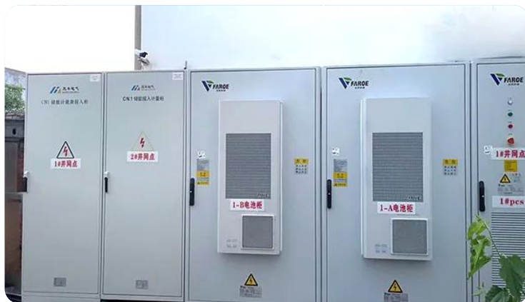
📍 Jiangsu Suzhou 400kW/1290kWh
