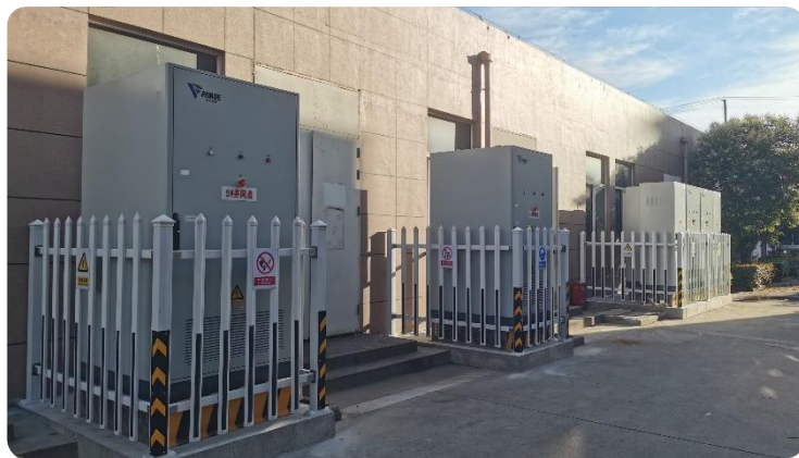
📍 Jiangsu Nantong 400kW/964kWh
