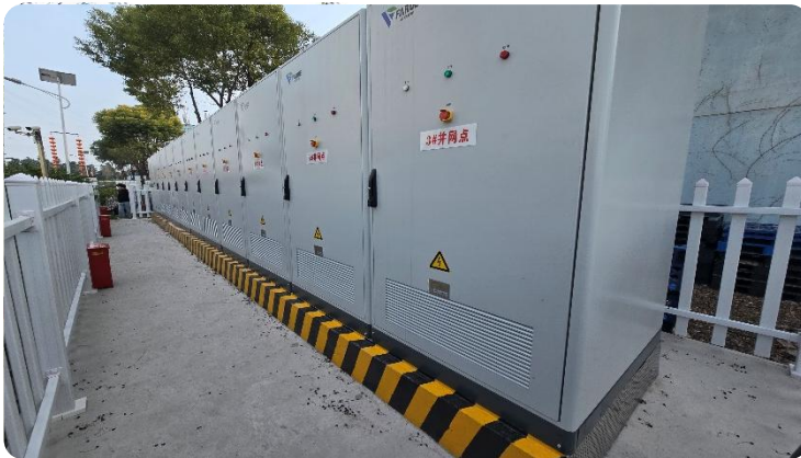
📍 Jiangsu Haian 1200kW/2580kWh
