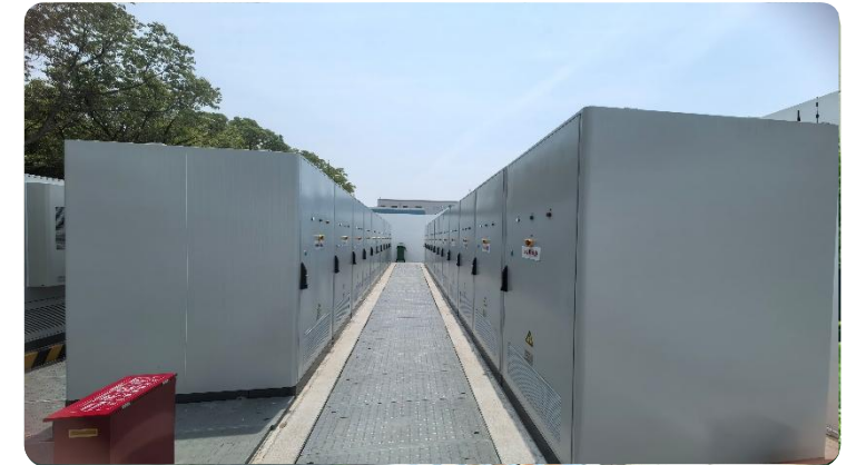
📍 Jiangsu Haian 5900kW/14219kWh
