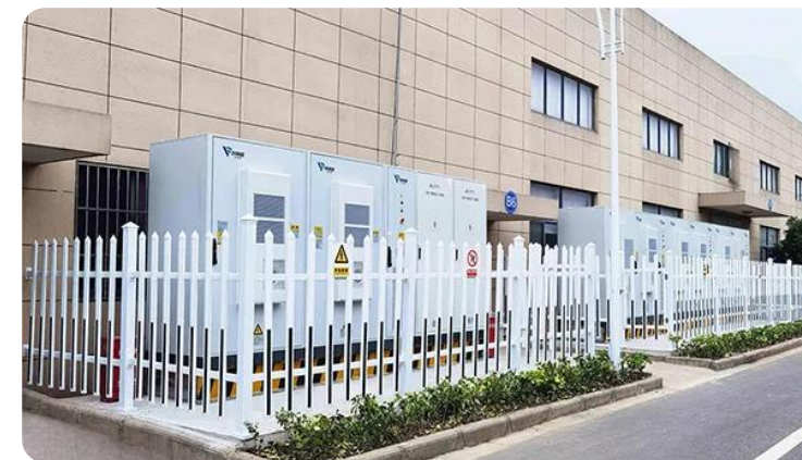
📍 Jiangsu Nantong 800kW/2580kWh
